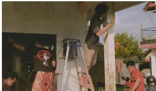
Figure 6. Activities peeling wall paint part outside and inside worn room
