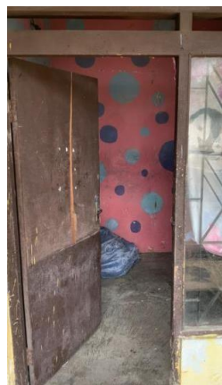
Figure 4. Condition of the Ronda Post Door
