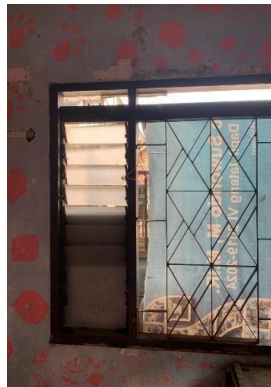
Figure 3. Condition of Window Glass Ronda Post
